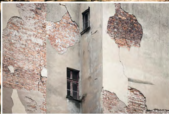
A new severe event of shrinkage and swelling of clay causes cracks on buildings.
